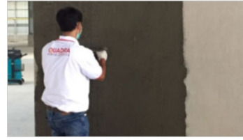
4.1.3 Apply the adhesive on the back of Quadra and on the wall, spread in one direction with adequate tile trowel
