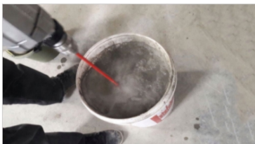
4.2.1 Mixed water and adhesive proportionally and use only adhesive class C2TES1 to get the best result
